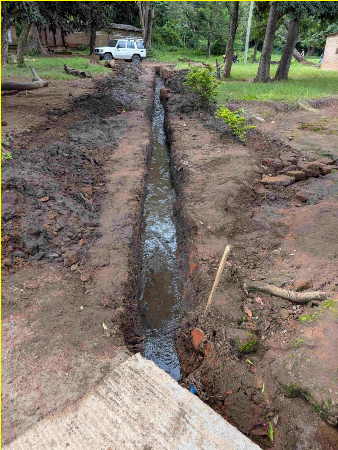
Ditches were dug where natural runoff occurs and replaced with perforated pipe and gravel and covered.
