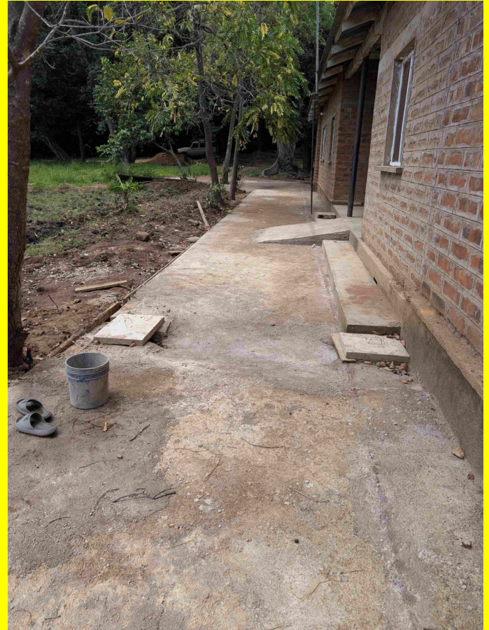
"Troubling" north side followed similar process as described to the left but covered by a solid concrete walkway.
