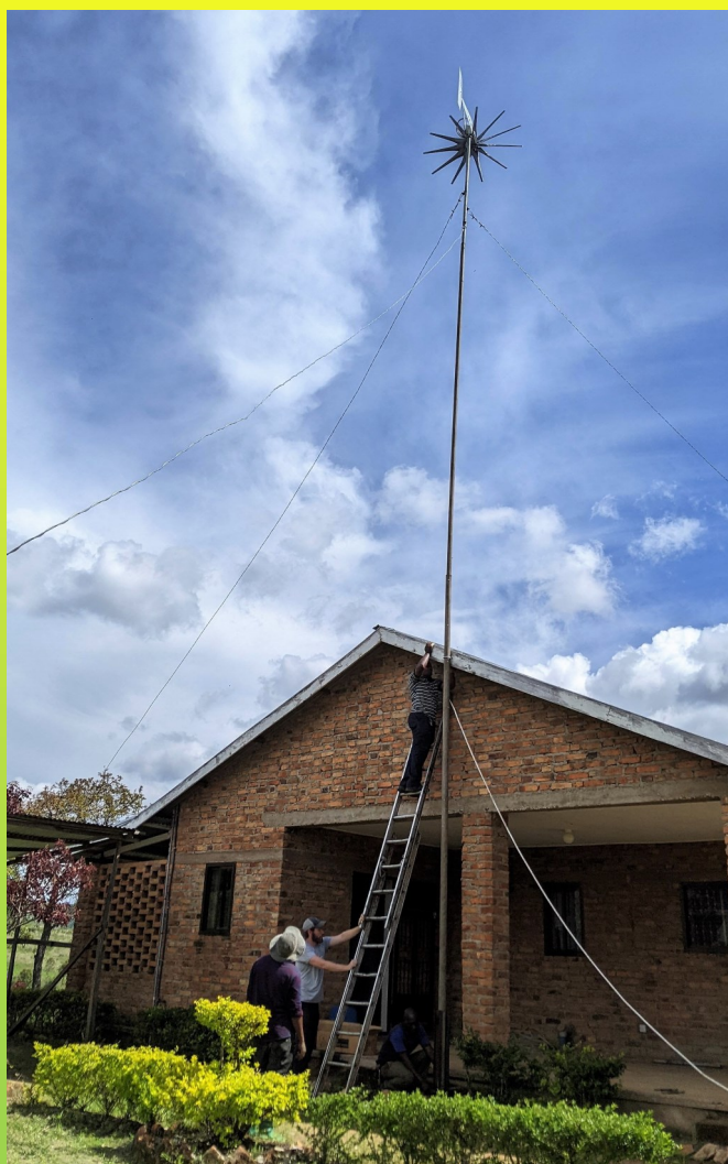
It has been eight years since Mary and I moved to Chimala to begin restoring the old Ailsa farm house to help re-establish that work which had been abandoned in the late 1970s. After a major setback, we have finally completed the off-grid electrical system as TANESCO does not provide power in that area. Finally there is now both solar and wind power adding both livability and security to the work at the Ailsa farm.
