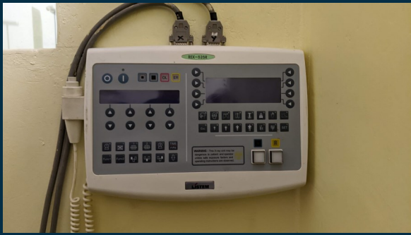
Display Console Needs Replaced
