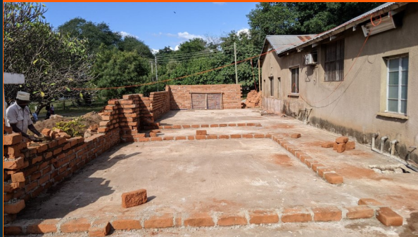
Foundation, exterior brick walls and floor plan in the beginning stages of construction.
